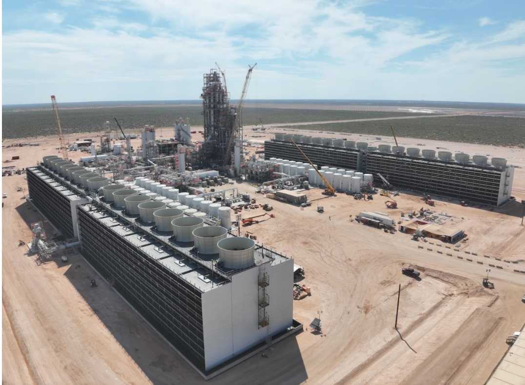
1PointFive's STRATOS Direct Air Capture plant
