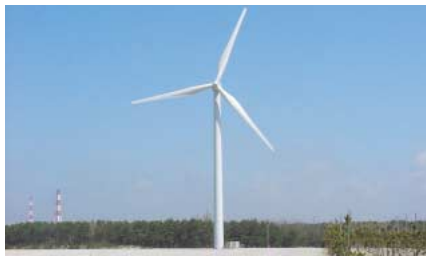
Wind power generation unit at the Akita Oil Depot
