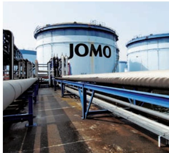
Storage tank and pipeline at the Keihin Delivery Terminal
