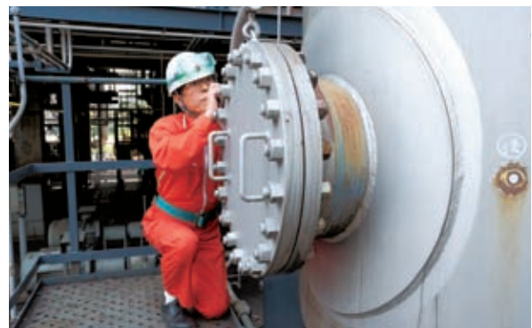
Inspection during a regular maintenance check
