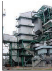
Flue-gas denitration equipment
