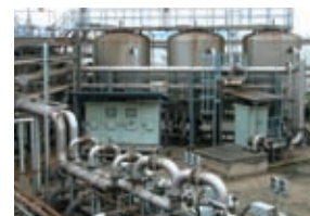
*2 Activated carbon absorption facilities
