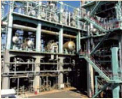
Ethylene manufacturing equipment at the Kawasaki Plant
