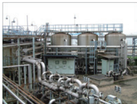
2: Activated carbon adsorption unit
